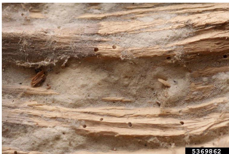
Wood damage from powder post beetles.
